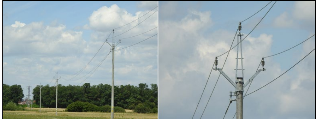
Fig. 3. For newly constructed lines, crossarms with side arms angled upwards are often used. This is both a long-lasting and a very effective measure. Photos from Raptor Protection of Slovakia.
