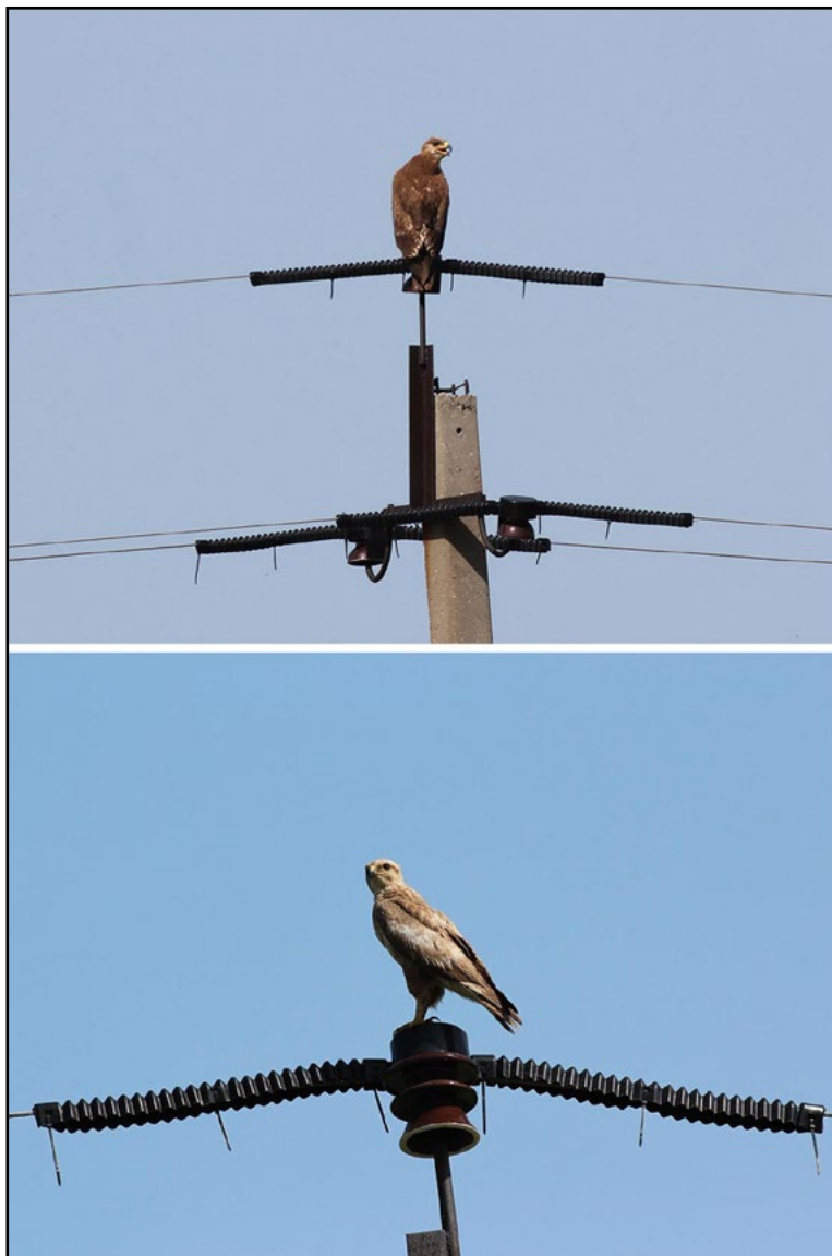
Steppe Eagle (Aquila nipalensis) and Common Buzzard (Buteo buteo) on power poles with bird-protective covers from the Eko-NIOKR company.
