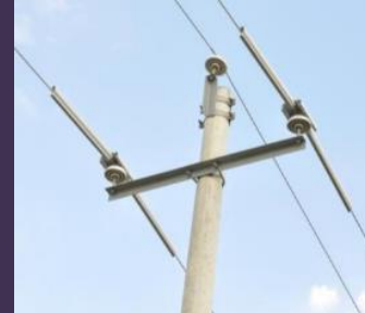
Insulation: on cables
