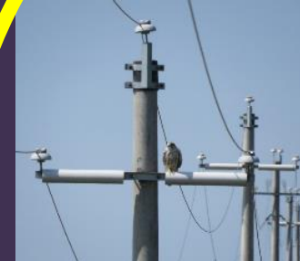
Insulation: on supports
